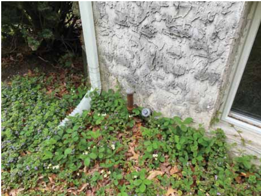
Photo 4: View of vent & fill pipes associated with a No. 2 heating oil AST situated in the basement of residence #1 onsite.
