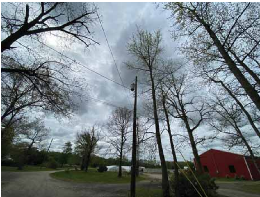
Photo 24: Representative view of an existing pole-mounted electrical transformer present on the Site.
