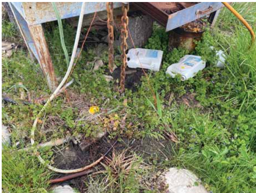
Photo 13: Representative view of the petroleum-based staining (REC-8) in the underlying vicinity of the two (2) diesel fuel ASTs pictured in photograph #12.
